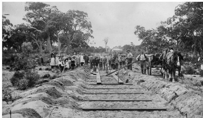
Making of plank road, Osborne Park, 1913-14 (courtesy of the Battye Library, State Library of Western Australia (3239B_61)). This image shows how a typical plank road was constructed.
